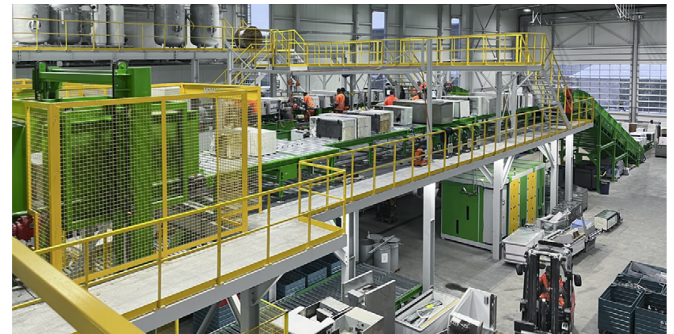
Erdwisch refrigerator recycling plant of Immark AG. Middle: upper plant deck with extraction stations, left: appliance infeed in the second processing stage, with the N2 production plant in the background.
