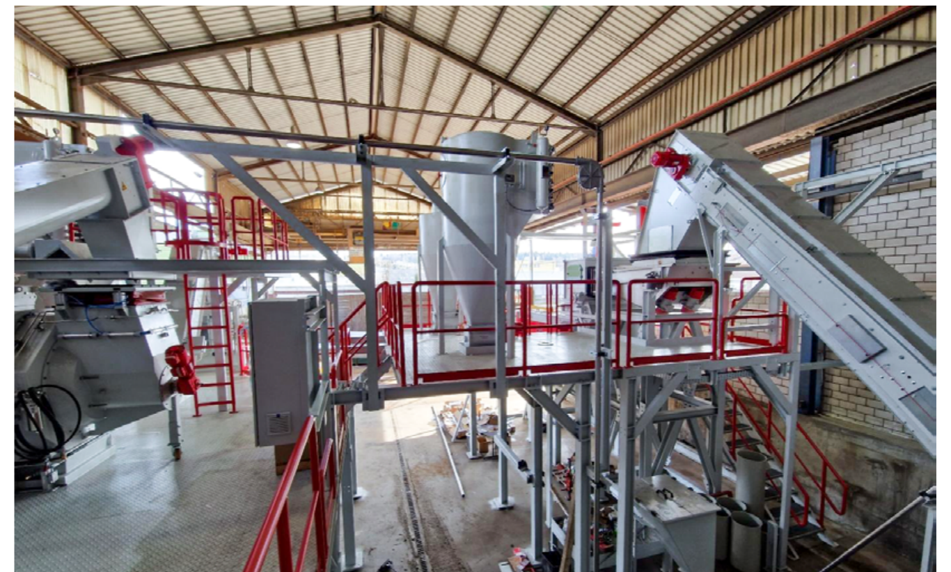
E. Flückiger AG refrigerator recycling plant from URT under construction. Left: pellet press, right: plastic/aluminium discharge belt on the eddy current plant.
