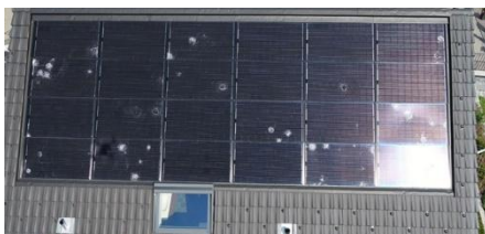
Figure 3: Drone image of a house roof with hail damage, copyright: Energie Netzwerk, Heinz Simmler.
